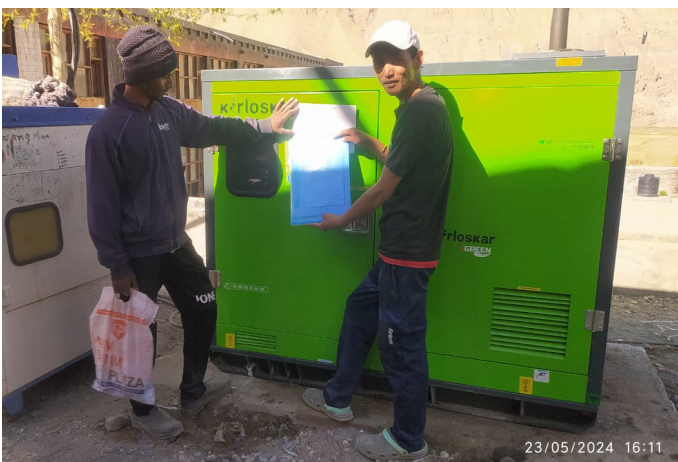
Our new electrical generator in operation at Munsel-ling
